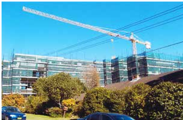
The apartments nearing completion – from our street outside our next-door neighbours' house
